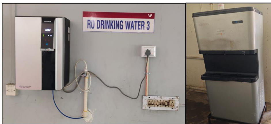
Water supply systems observed in the Campus
