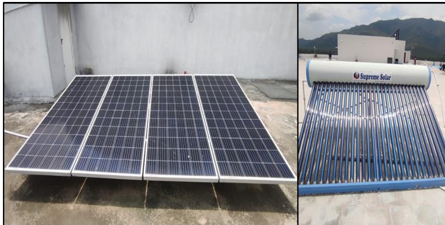
Solar Water Heater observed in the campus
