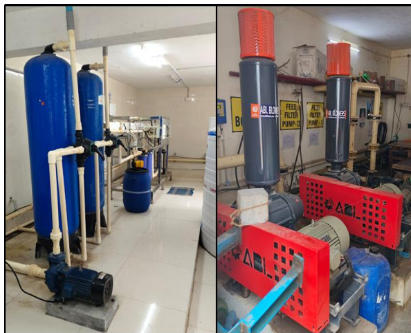
Sewage treatment plant observed in the Campus
