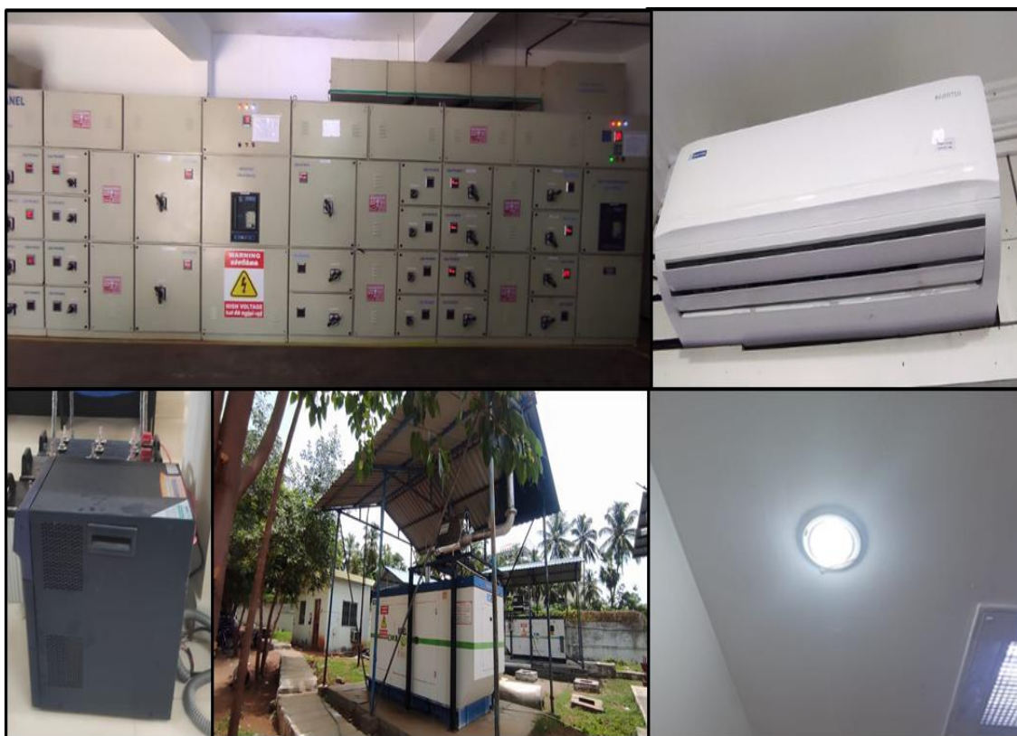
Energy conservation facilities observed in the Campus
